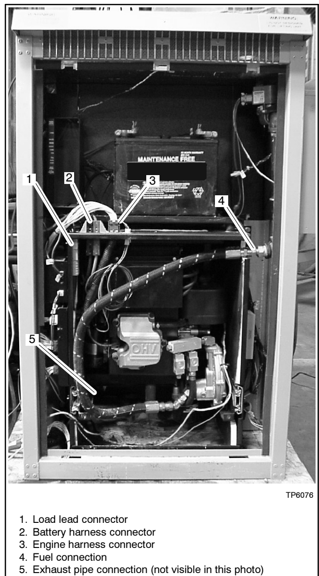
Figure 3-3 Generator Set Installed in Cabinet (door and front panel removed)
