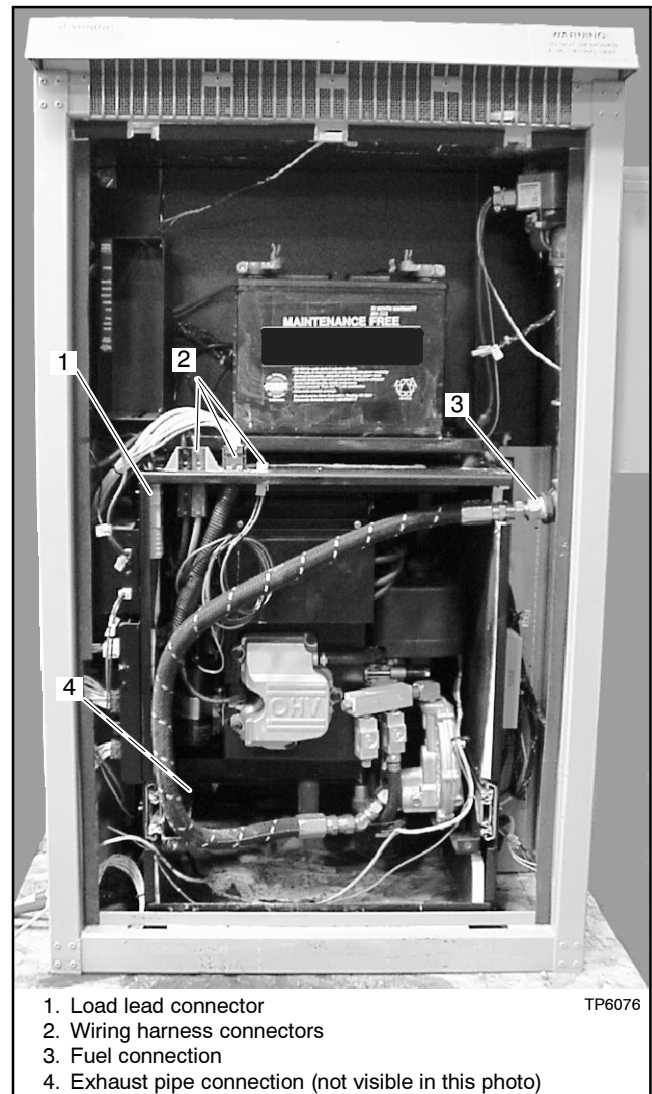
Figure 7-1 Generator Set Installed in the cabinet
